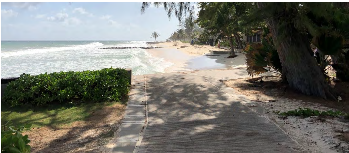
Figure C.12. Recreational area on Sir Richard Haynes Boardwalk – a successful example of a climate-resilient structure that is designed to reduce flooding impacts whilst increasing the accessibility to the coast.
